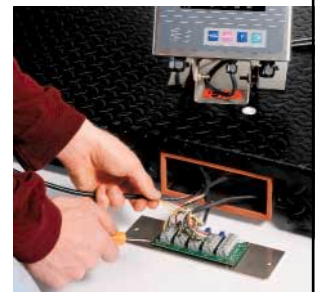
Simple access to J-Box wiring.
